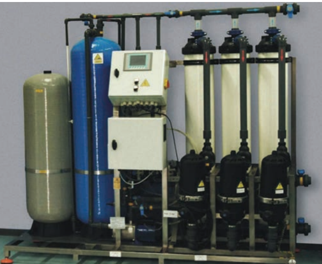
Water UF pre-treatment plant
